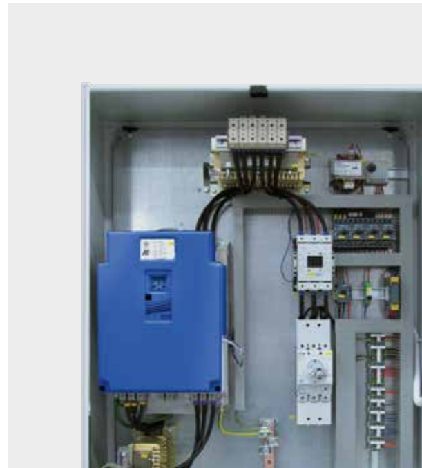
Standard or customised – power supply panels from AERZEN ensure the perfect motor start
