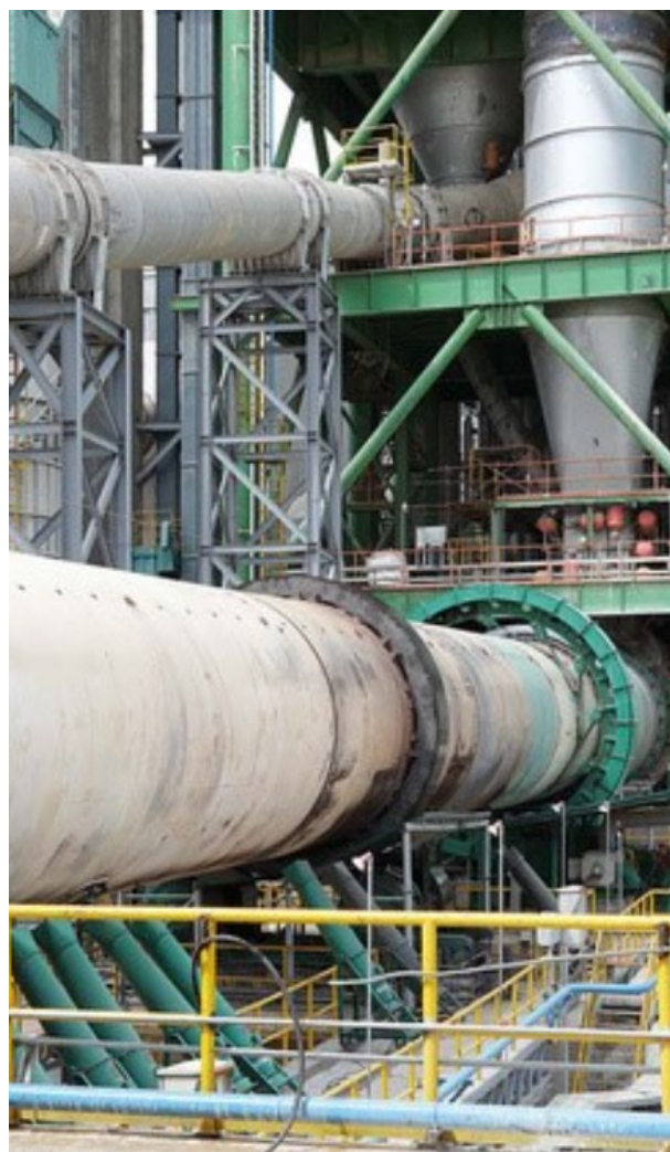
The burning process in the rotary kiln accounts for 90% of the total energy demand of a cement plant.
