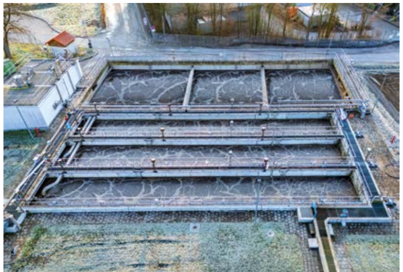
The biological treatment stage comprises two aeration tanks. The first is flowed through in three cascades connected in series, while the second is divided into three channels operated in parallel.
