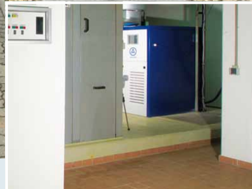
Besides a positive displacement blower series DELTA BLOWER, which extracts exhaust air and feeds it into the aeration basins, wastewater treatment plant Arnsberg-Wildshausen also has a new Aerzen turbo blower in the central compressed air station.
