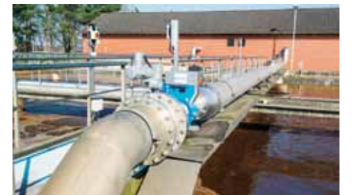
With diaphragm regulating valves and modified speed the air introduction into the tanks is controlled.
