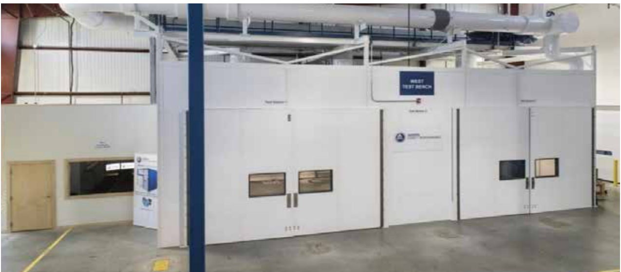
Overall view of ASME PTC 13 conforming factory test facility at Aerzen Coatesville facility.
